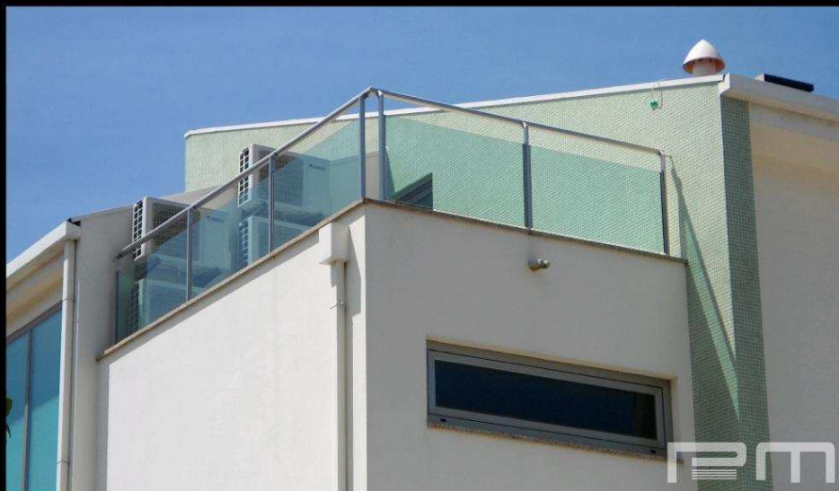
Aço Inox e Vidro . Stainless Steel and Glass
